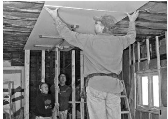
Dave Reichard, Jim Jones and Roger Forden install drywall on a ceiling at a Habitat house near MLK Park
